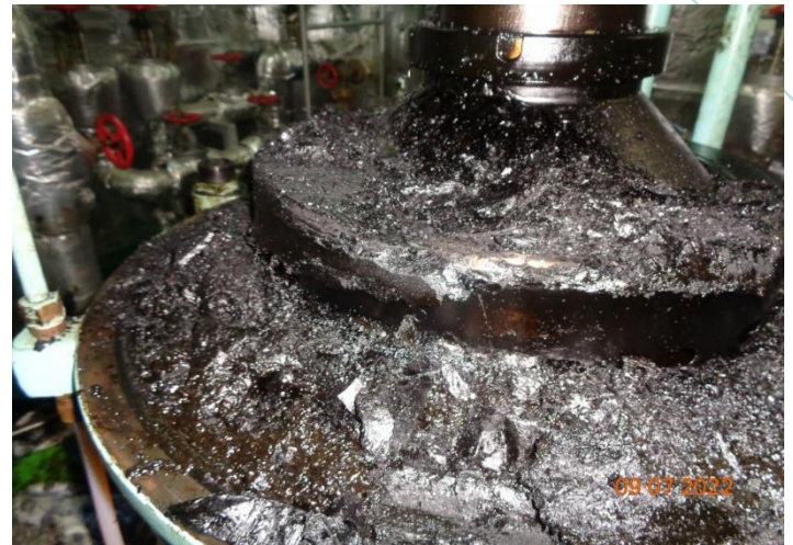
A purifier fouled with hard excessive asphaltene sludge
